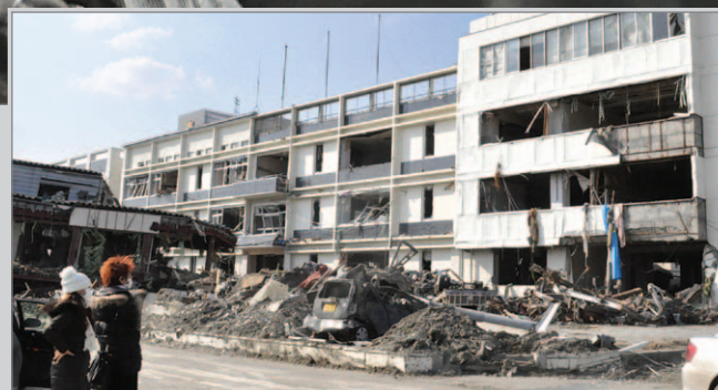
Tsunami waves reached the third floor of Rikuzentakata’s City Hall building.
